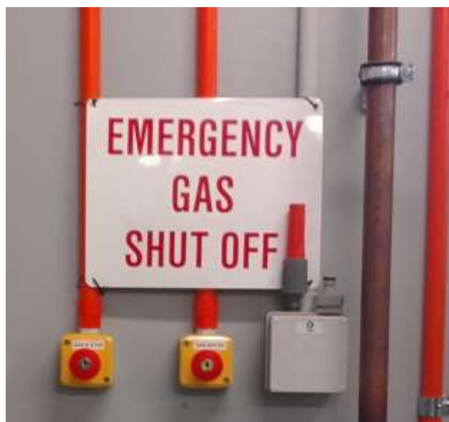
Figure 5: Emergency gas shut off system located in the Gas Laboratory (Figure 3).
