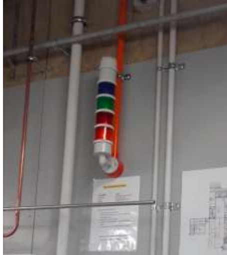
Figure 4: Gas Alarm system, located in the Gas Laboratory (Figure 3). The lights will alert to type of emergency.
