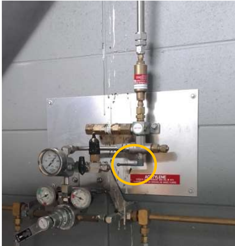
Figure 6: Acetylene shut off valve (Location: Figure 3). To shut off position grey lever (circled) to a 90° angle to its current position if safe to do so .
